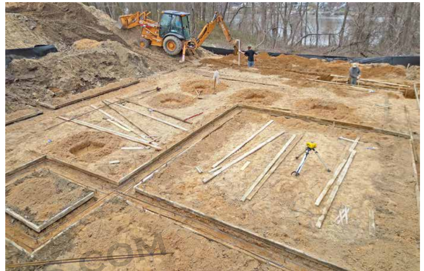
Figure 3-1. Excavation for foundation footings. The soil has been excavated and flattened to bring the entire lower floor below the frost depth. Trenches are then dug for the footings. In this loose soil, the trenches are lined with boards. Steel reinforcing rods are supported within the trenches to strengthen the footings. In addition, five holes have been dug to act as forms for individual footings for columns that will support the interior structure of the house. DRW
