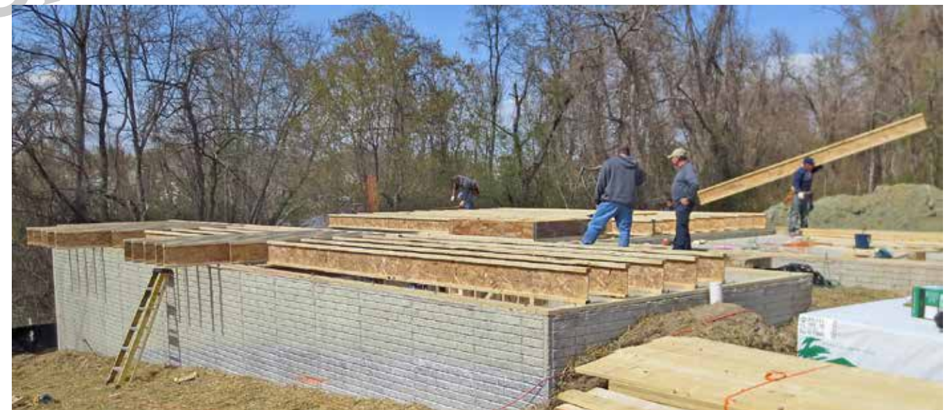
Figure 3-17. The floor joists being installed on the foundation. The outer ends rest on the sill plates. The inner ends rest on beams and/or load bearing walls that were built as interior parts of the foundation. These floor joists are made of composite “I-joist” material, which is now prevalent. However, some houses still use the older style of solid timbers, which have both advantages and disadvantages. DRW
