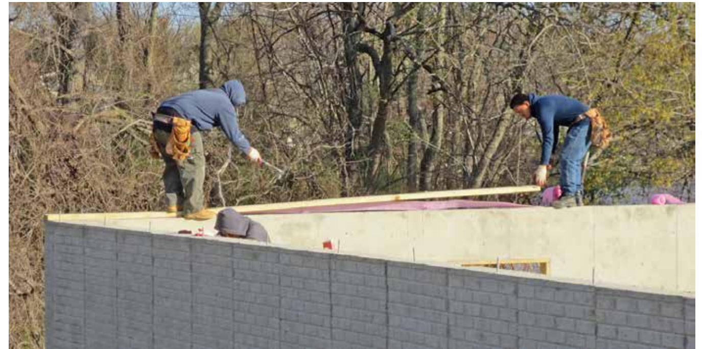
Figure 3-16. A “sill plate” being installed on the foundation. This is the first step in platform frame construction. The sill plate is anchored to the foundation with bolts that are embedded in the concrete. The pink strip between the sill plate and the foundation is “sill sealer.” It prevents air leakage through the gap between the lumber and the concrete. DRW
