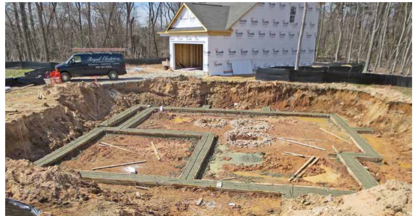
Figure 3-2. Completed footings. Grooves along the centers of the footings act as keyways to prevent the foundation walls from being pushed off the footings by soil pressure. This foundation also has four individual footings to support interior columns. Only one was poured when the picture was taken. DRW
