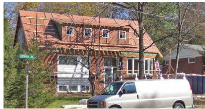
Figure 1-126. Increasing the roof slope to convert a low attic into living space. The house to the right shows the original slope.
