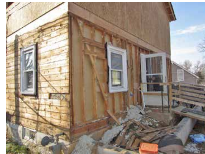
Figure 1-127. Adding a second story to a house that has frame walls. The original board sheathing of the exterior walls is being replaced with plywood sheathing for additional strength. This modification is in the wrong sequence. The lower walls should have been strongly reinforced before adding the second story.
